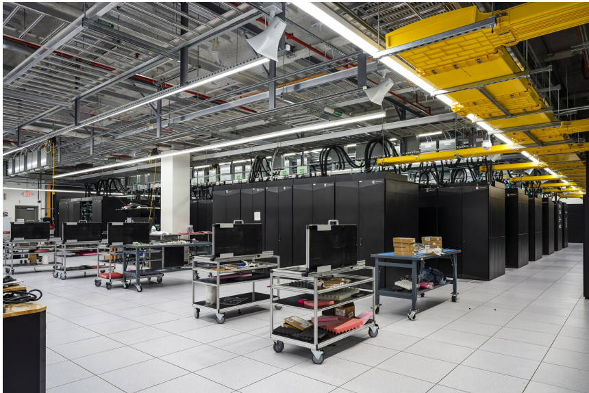
The Frontier supercomputer at Oak Ridge National Laboratory, photographed in July 2022. The equipment floor shows the physical systems behind large-scale computation. Photo: Oak Ridge National Laboratory, CC BY 2.0, via Wikimedia Commons .
